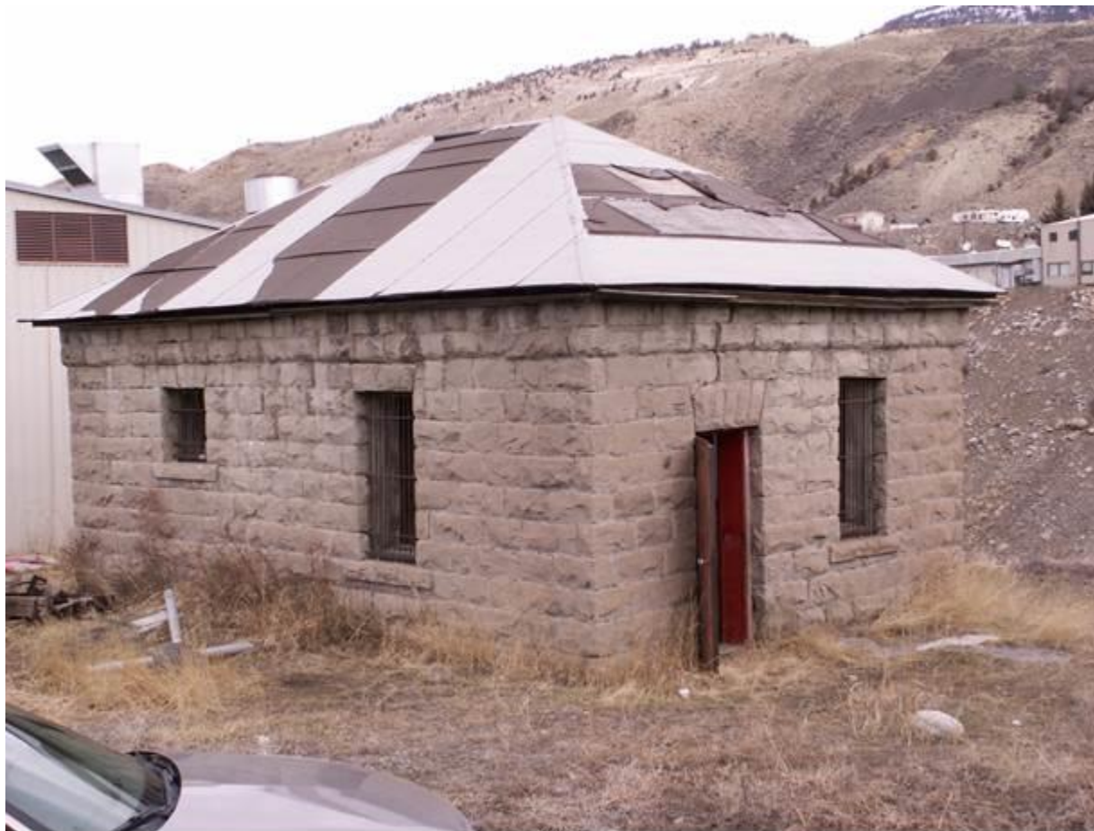
Description and view of camera: East and South elevations, view to northwest
