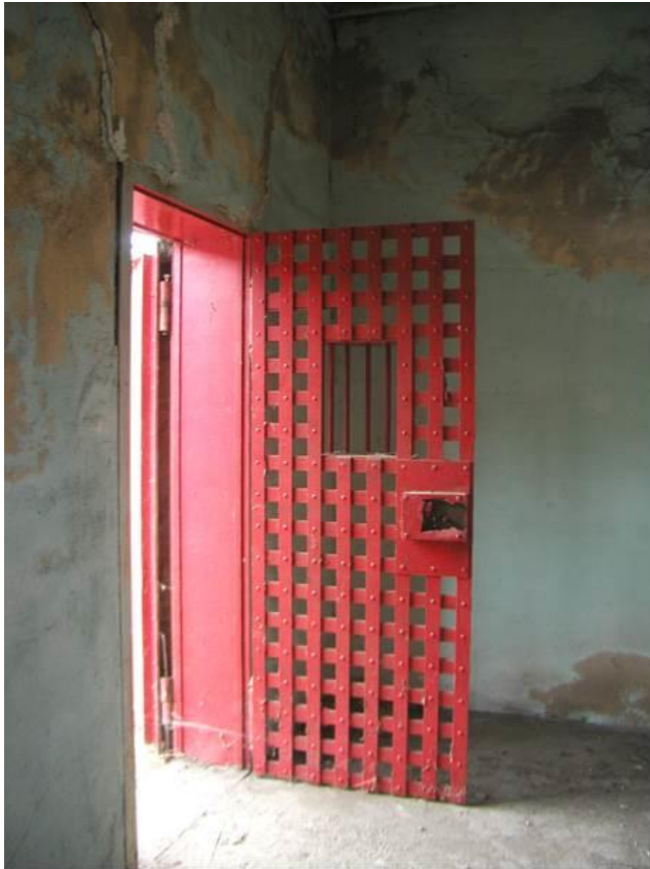
Description and view of camera: Interior entry door, view to southeast Photograph: MT_ParkCounty_GardinerJail_0009
