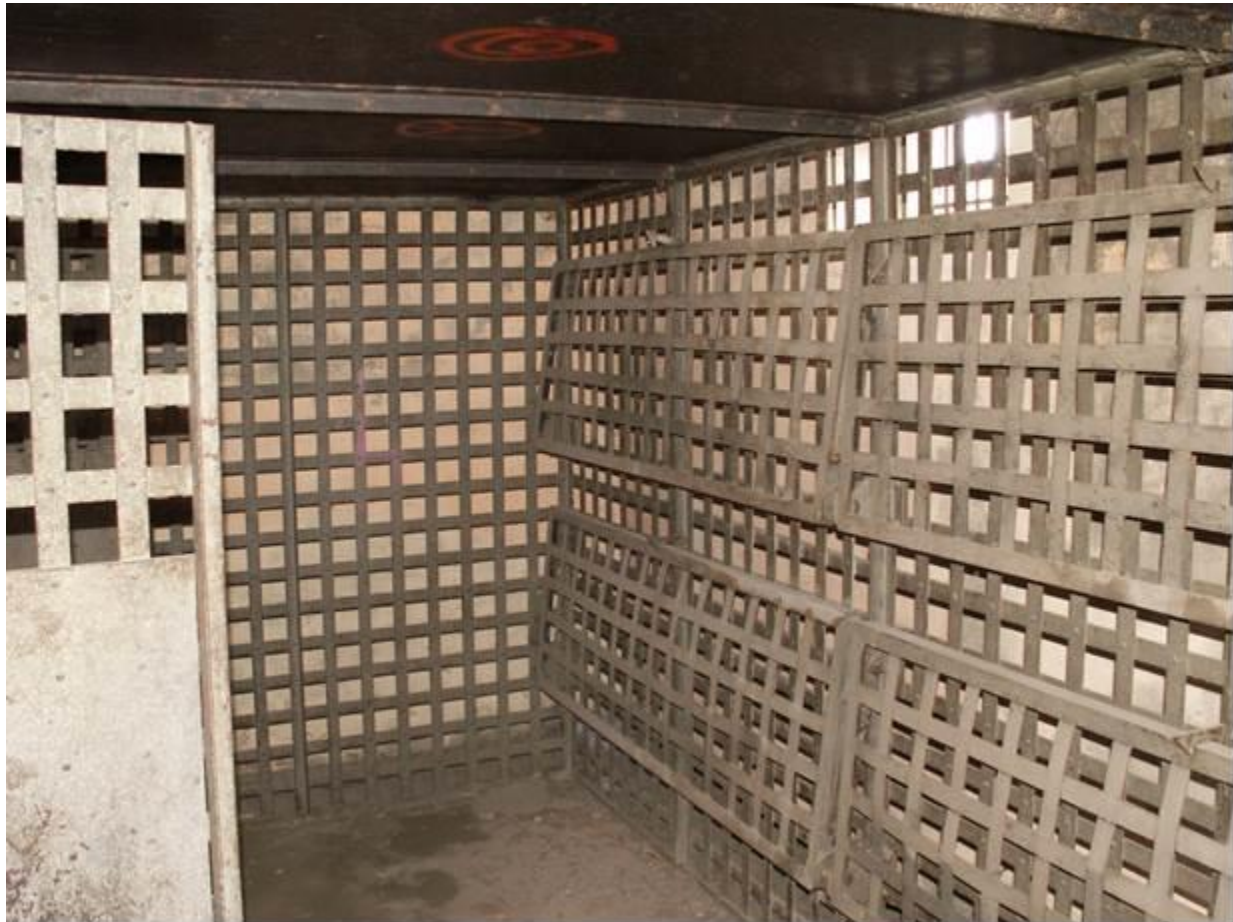
Description and view of camera: Interior, four-person cell, view to west Photograph: MT_ParkCounty_GardinerJail_0008
