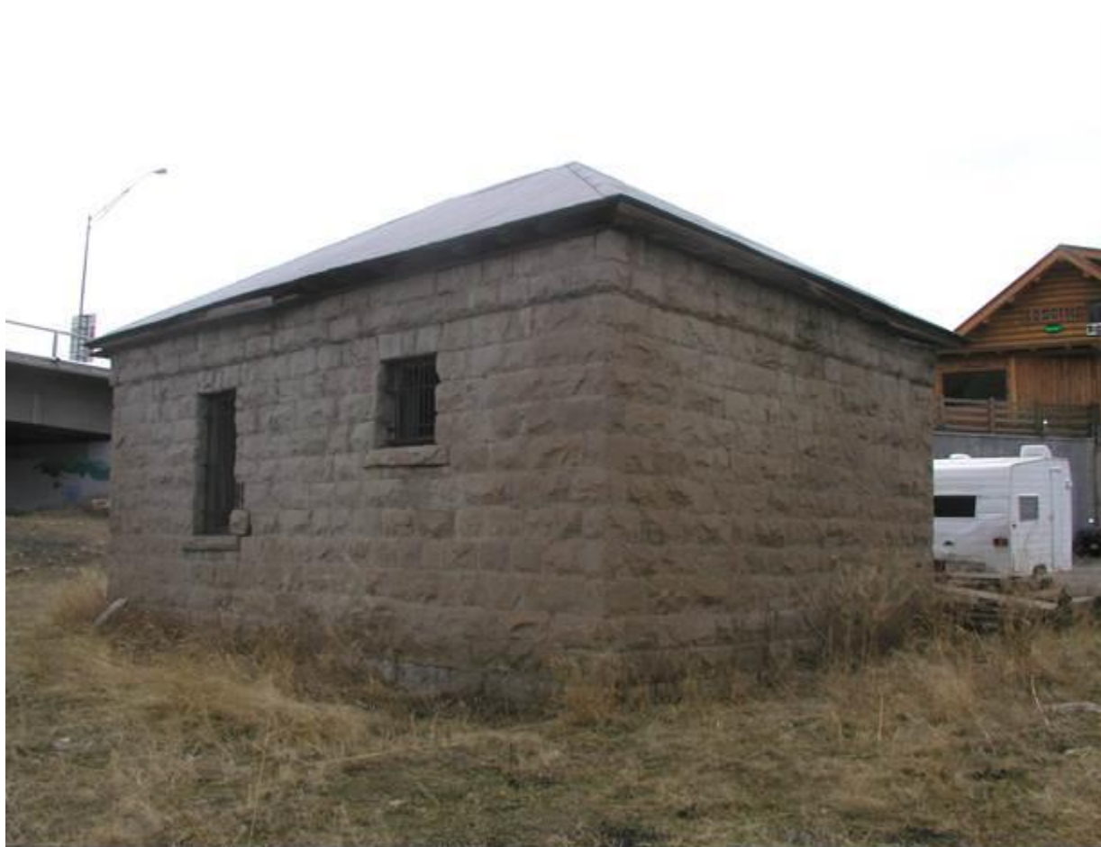
Description and view of camera: North and West elevations, view to southeast Photograph: MT_ParkCounty_GardinerJail_0004
