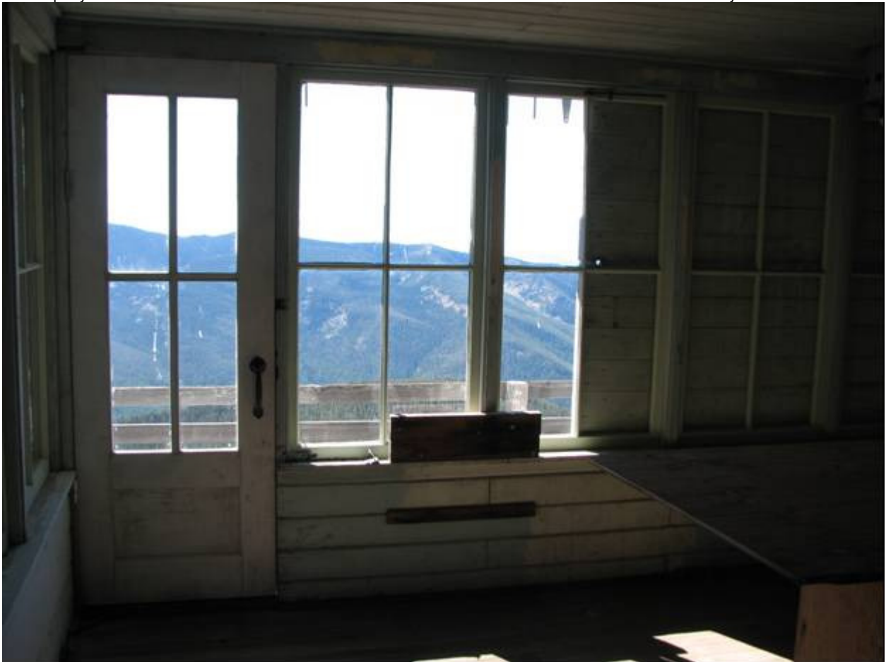
MT_MissoulaCounty_MineralPeakLookout_0005. Looking south to the front wall of the lookout house from the interior.
