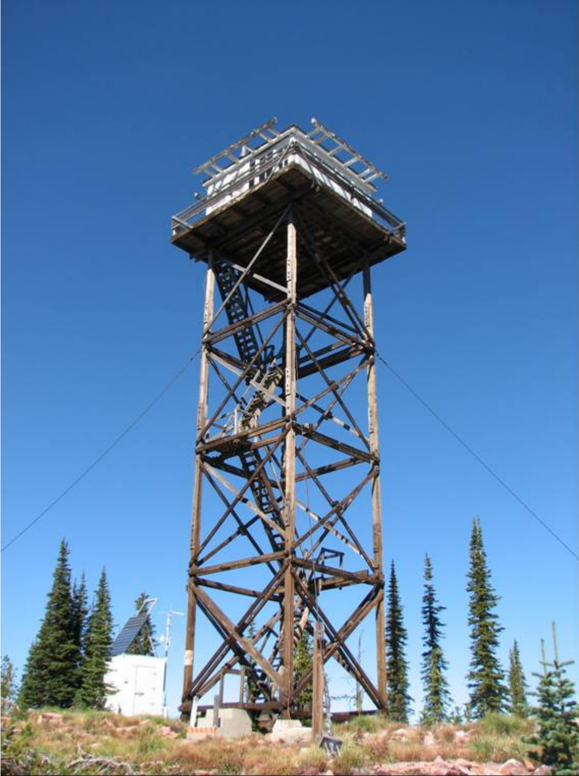
MT_MissoulaCounty_MineralPeakLookout_0003. Looking northwest to the south and east sides of Mineral Peak Lookout. The radio relay and weather station visible in left of photo.
