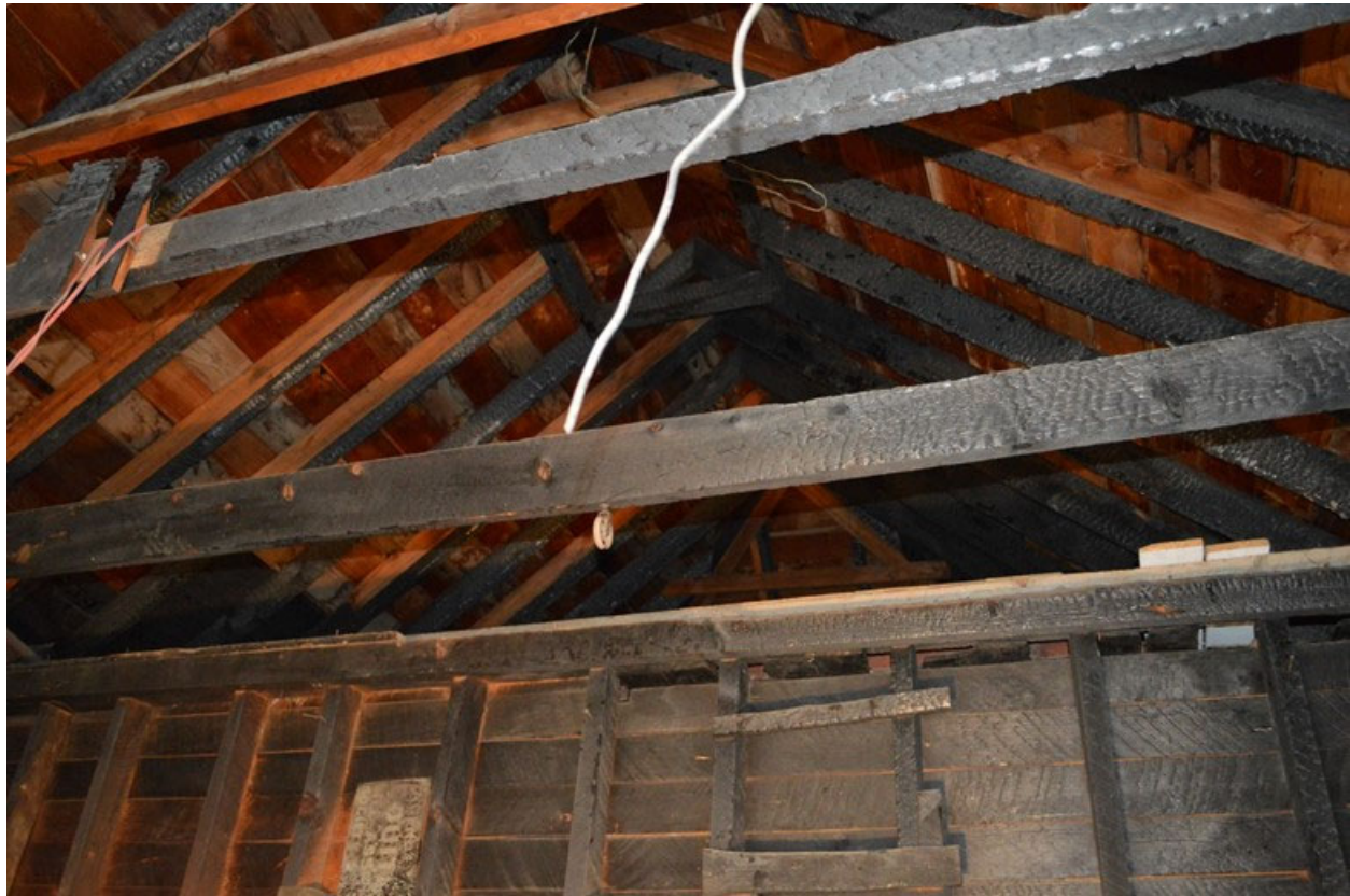
MT_LewisAndClarkCounty_Shaw'sBestFactory_0007 of 0020: Shaw's Best Factory. Second floor interior burnt rafters and adjacent replacements from the 1933 fire.
