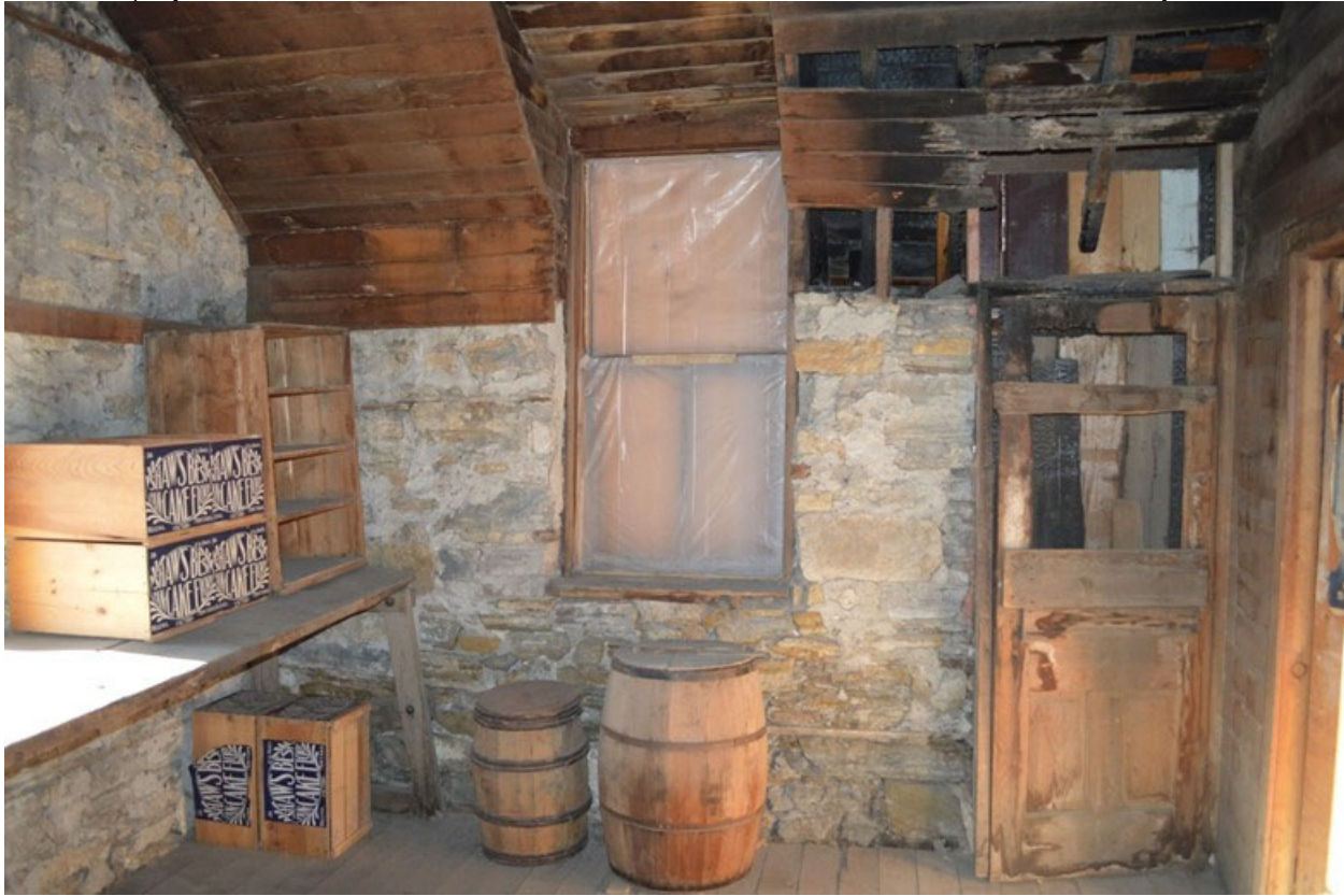
MT_LewisAndClarkCounty_Shaw'sBestFactory_0010 of 0020: Shaw's Best Factory. Second floor interior, west residential/production room, looking west at pedestrian entry.
