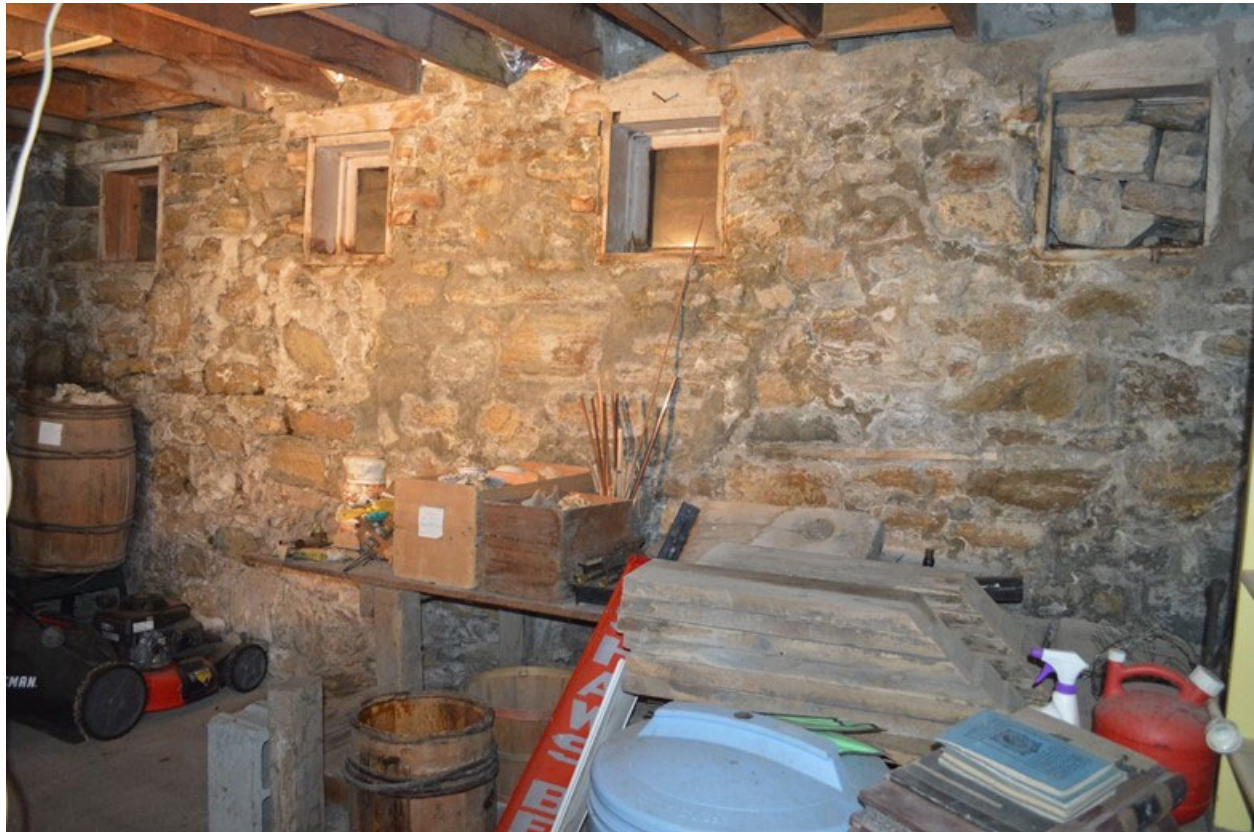
MT_LewisAndClarkCounty_Shaw'sBestFactory_0006 of 0020: Shaw's Best Factory. First floor interior north wall, horse stall windows, looking northwest.
