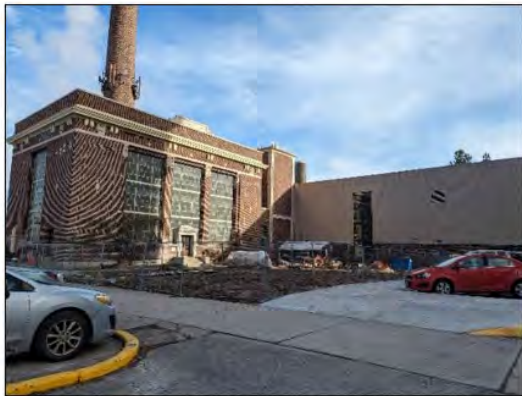
South Façade of existing heating plant and west façade of new CHP. February, 2024.
