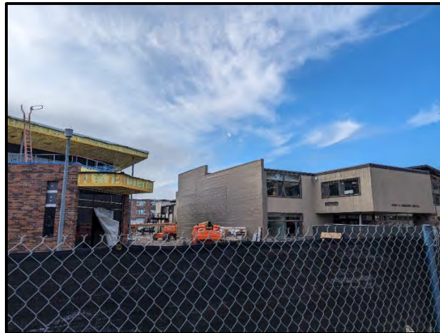
East side of Emma B. Lommasson Center (right) where it was demolished and sealed. Portion of new dining facility (left), February 2024. Due to construction footprint and fencing it was not possible to get a current picture of Craig Hall. Photo: Nikki Manning
