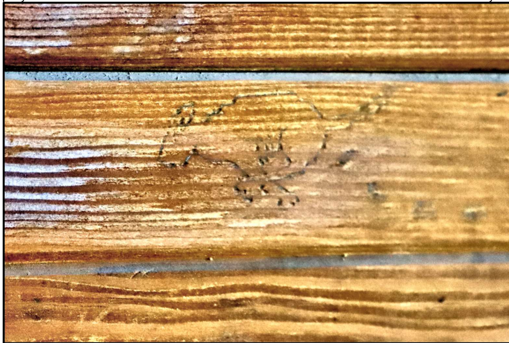
Photo 18: MT_WheatlandCounty_JudithGapJail_0018. View of wall A3 with a pencil drawing of a running rat. View direction north in 2025. (Photographer: Tim Urbaniak)
