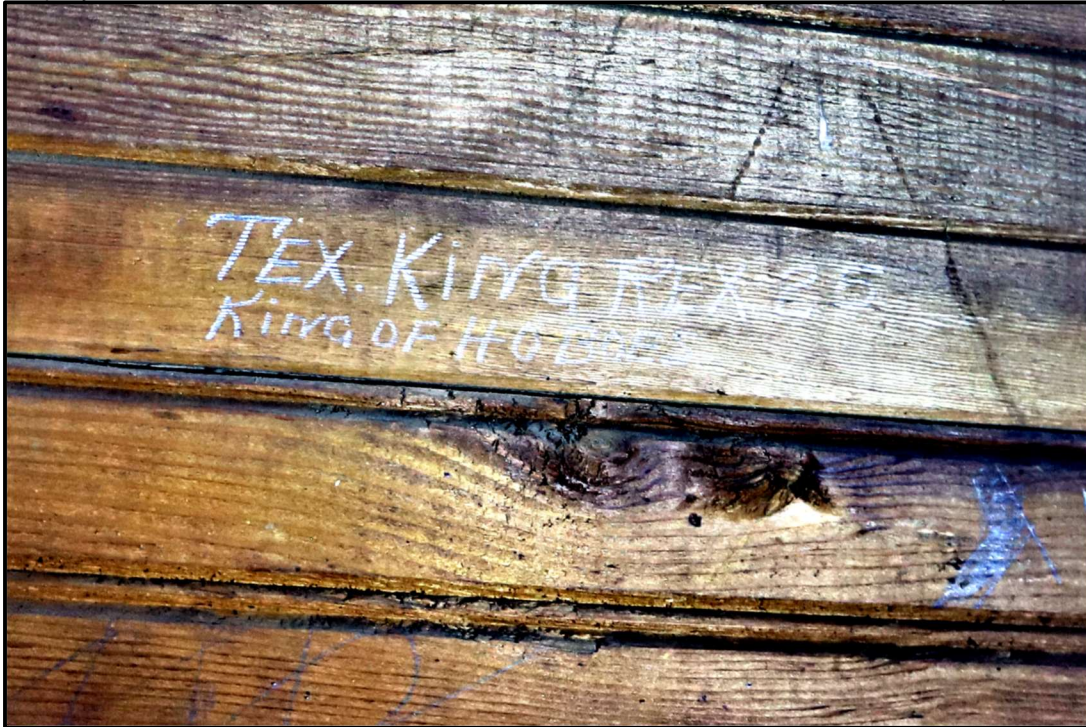
Photo 24: MT_WheatlandCounty_JudithGapJail_0024. View of wall A4 with the inscription of "Tex. King Rex 26. King of Hoboes." View direction north in 2025. (Photographer: Tim Urbaniak)
