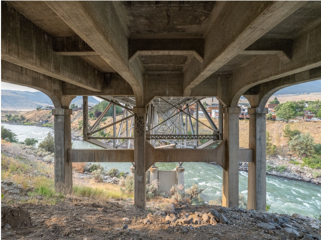
Gardiner Bridge. Detail of north approach span. View to the south. MT_ParkCounty_GardinerBridge_0015.
