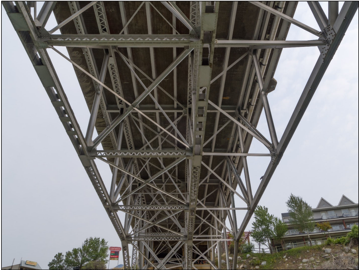
Gardiner Bridge. Detail of underside of truss. View to the north. MT_ParkCounty_GardinerBridge_0014.
