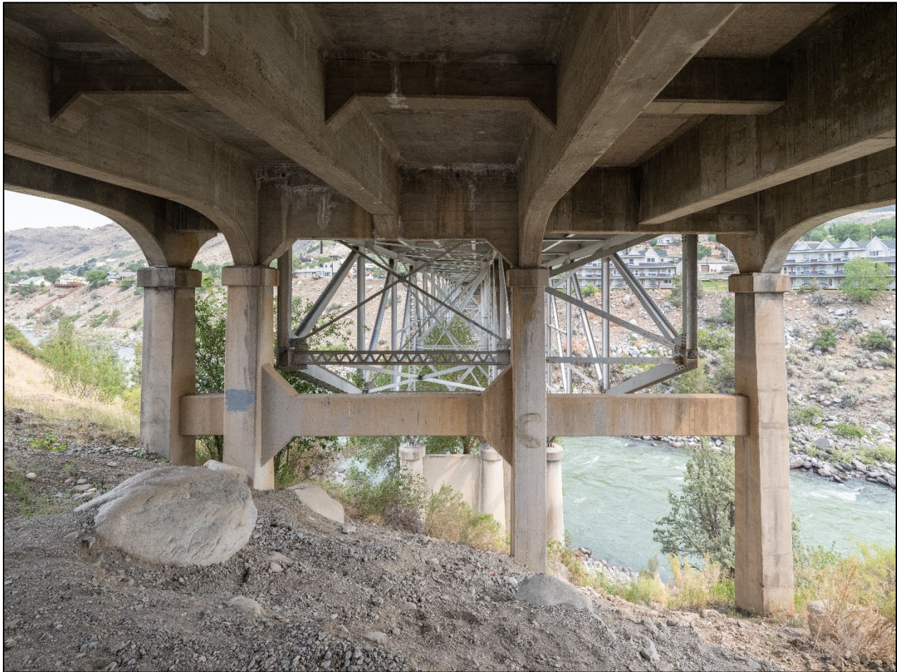
Gardiner Bridge. Detail of south approach span and truss. View to the north. MT_ParkCounty_GardinerBridge_0011.
