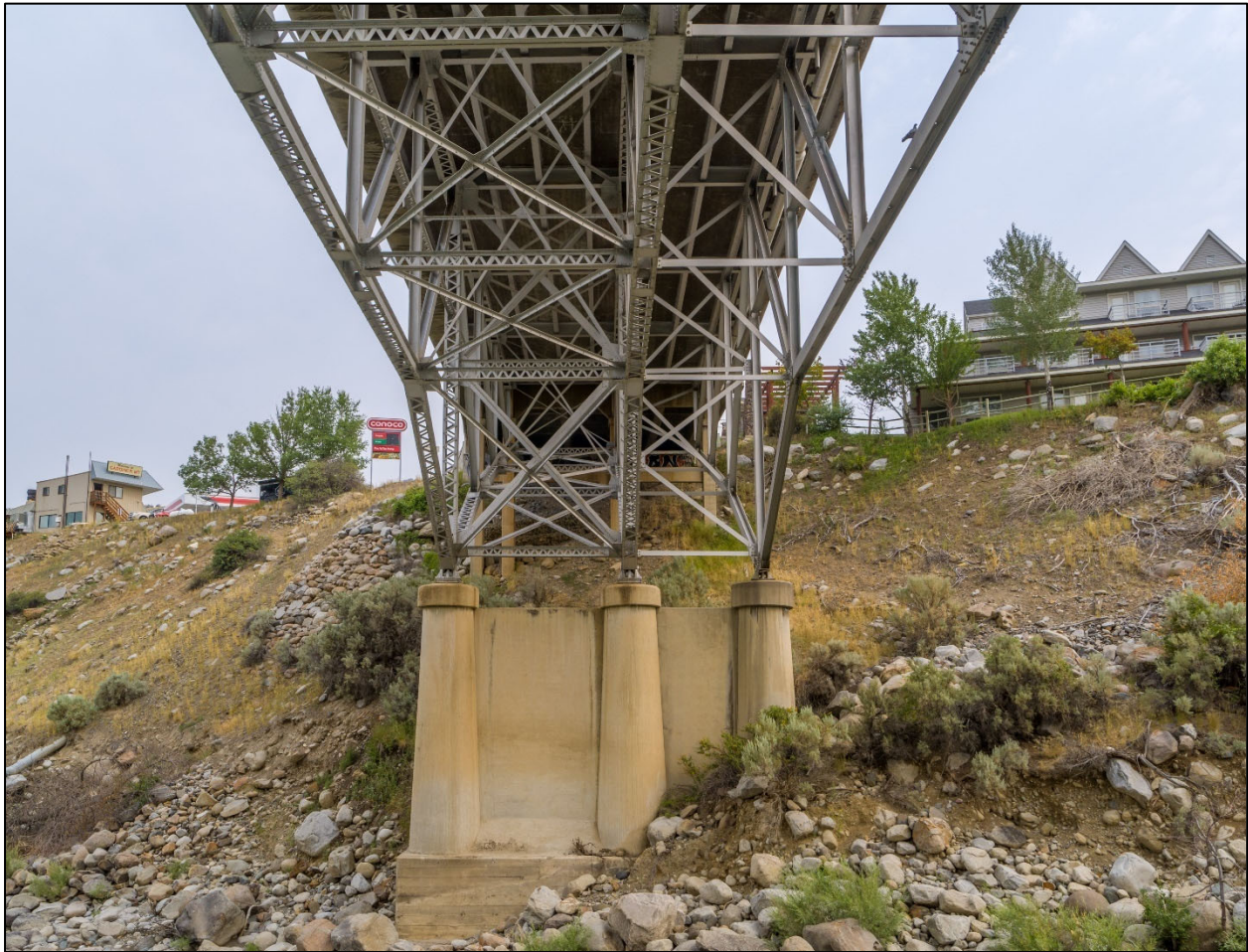
Gardiner Bridge. Detail of concrete bent and underside of truss. View to north. MT_ParkCounty_GardinerBridge_0013.
