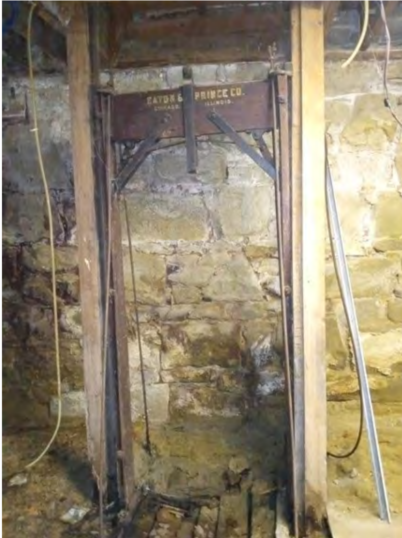
Basement of Farmers Trading Company showing close-up of elevator conveyance, view to North
