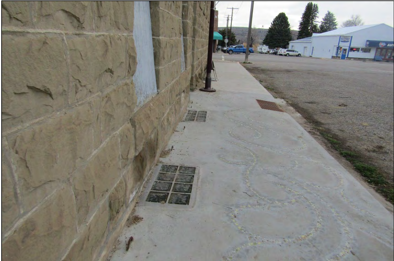
Farmers Trading Company. Detail of south side sidewalk blocks. View to the east. MT_CarbonCounty_FarmersTradingCompany_0012.
