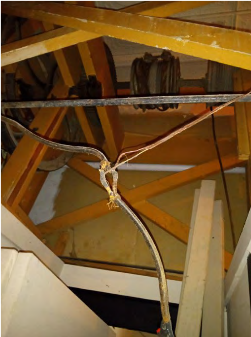
Main Floor of Farmers Trading Company, elevator hoist pulleys
