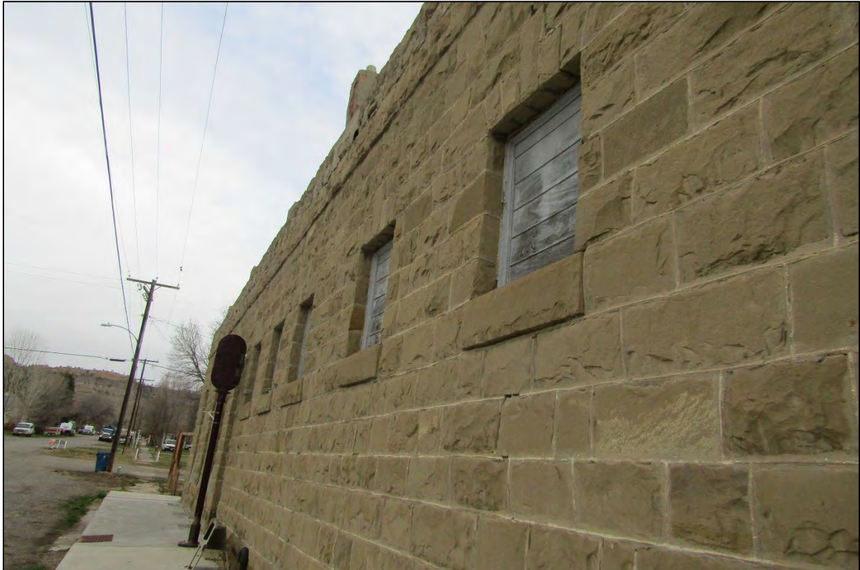
Farmers Trading Company. Detail of south side. View to the northwest. MT_CarbonCounty_FarmersTradingCompany_0010.
