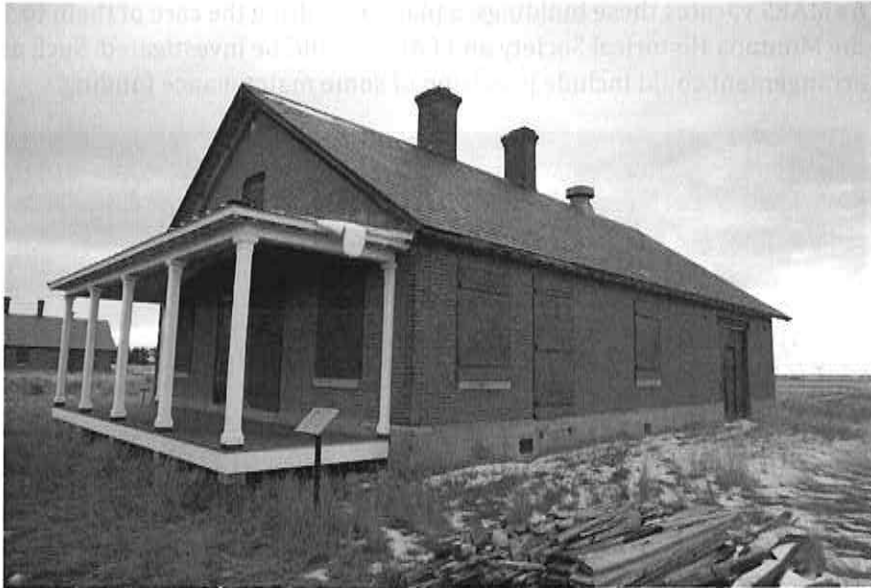
Figure 24: Double Cavalry Stable Guard/Shop #11, with new roofing and a rehabilitated front porch. Photograph taken January 22, 2020.
