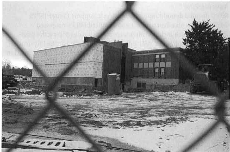
Figure 16: MSU-Billings Science Building's addition under construction; view from the southeast. Photograph taken January 12, 2020.
