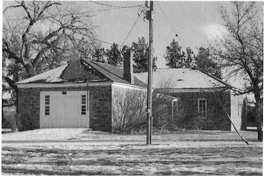
Figure 23: MAES Fort Assiniboine, Officers' Amusement Hall (Res. #6), as maintained in fair condition by FAPA. Photograph taken January 22, 2020.
