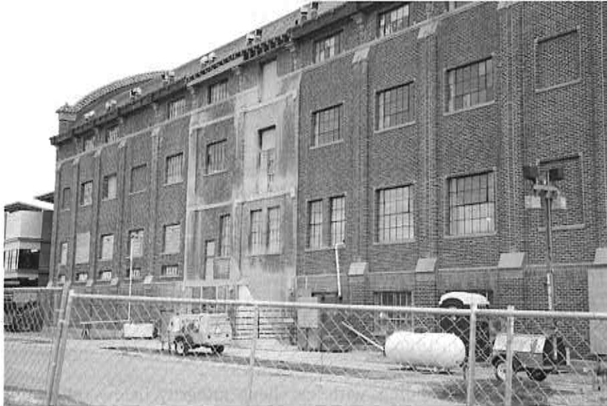
Figure 5: Romney Gym, showing where the original south stairs and enclosure have been removed. Photograph taken January 26, 2020.
