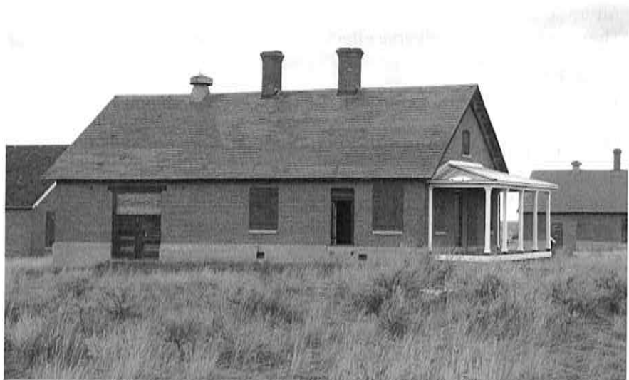
Figure 8: Fort Assiniboine's Double Cavalry Stable Guard and Shop (Res. 11), constructed in 1905. Both the slate roofing of the front gable roof and the standing seam metal of the front entry porch roof were replaced. Double Cavalry Stable Guard and Shop (Res. 12) is visible in the background. Photograph taken January 22, 2020.
