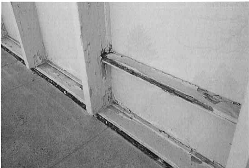
Figure 13: MSU's Northern gymnasium - close-up of rotten wood at south curtain wall. Photograph taken January 23, 2020.
