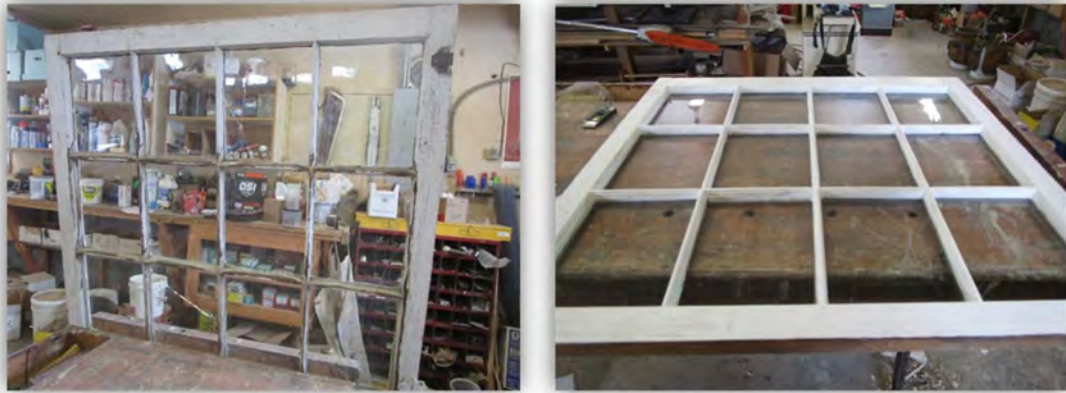
Repairing historic windows is a never-ending maintenance task for the preservation crew
