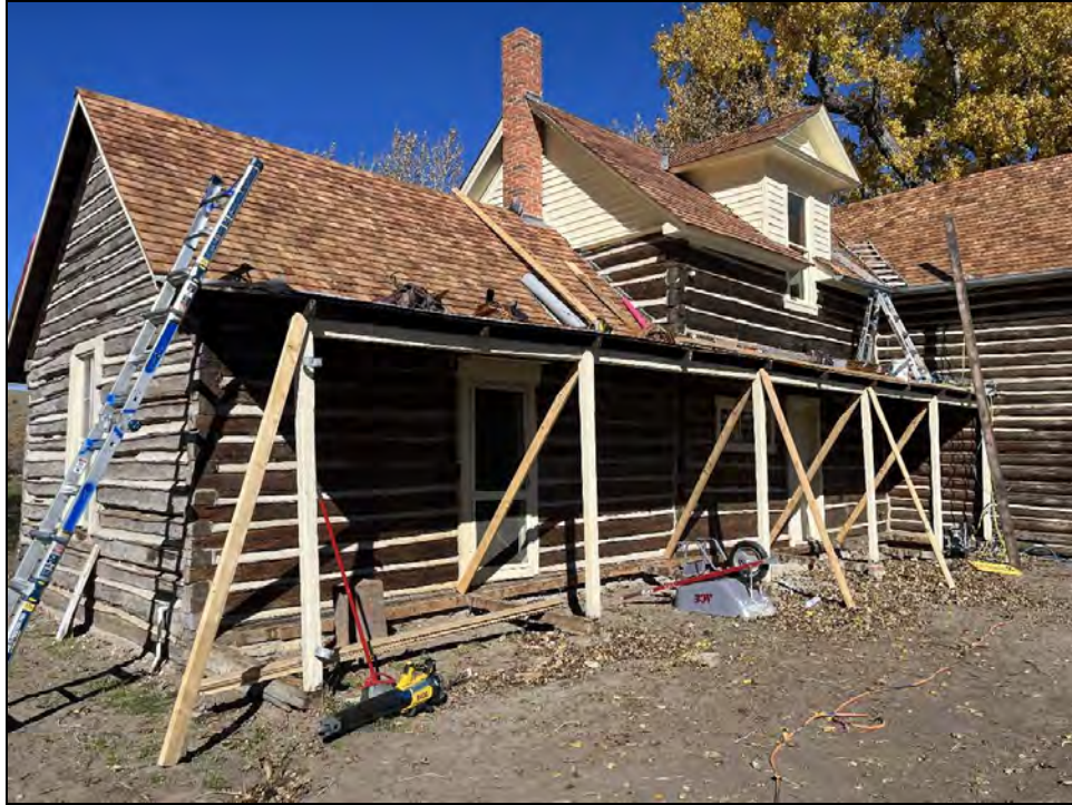
Figure 41. Before winter arrived at the end of October, the house was re-shingled, and the buildings secured against weather.
