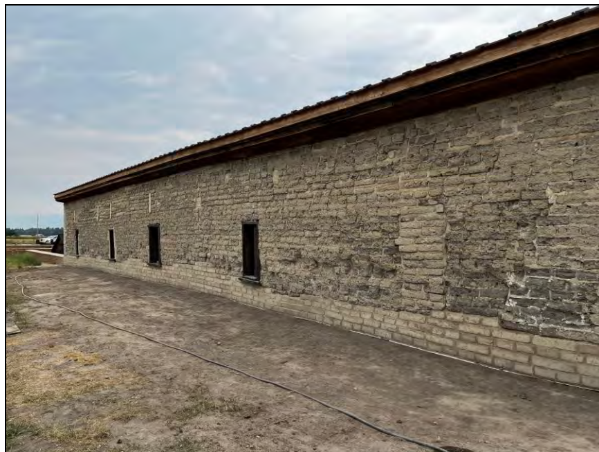
Figure 23: Completed adobe preservation on the East Wall of the East Barracks, originally built in 1857. Masonry preservation and new adobe fabrication by Zoula Masonry, LLC.
