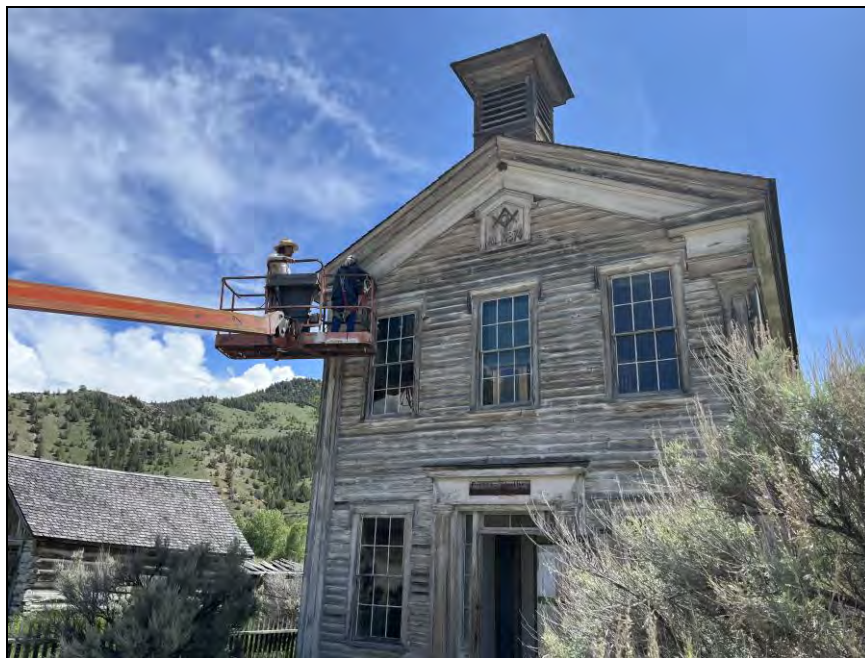
Figure 26. Architect Lesley Gilmore collects paint samples from the Masonic Temple while FWP maintenance staff member, Mike Kirsh, operates the hydraulic lift.
