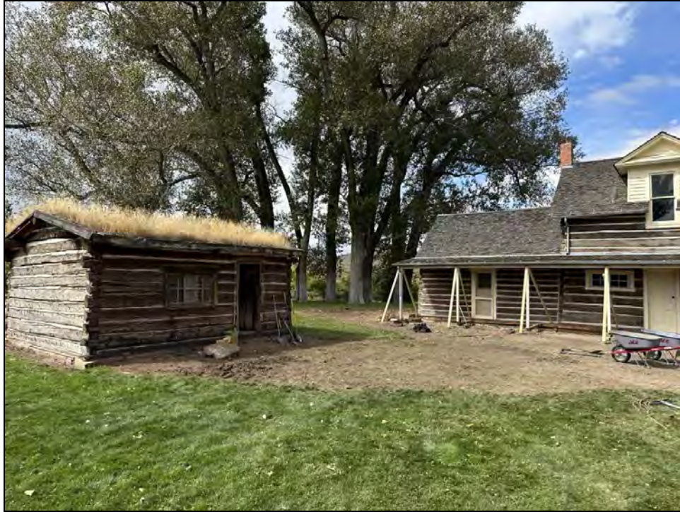
Figure 36. Overview of grading around Chief's House and Store. Selective demolition of porch is also evident.
