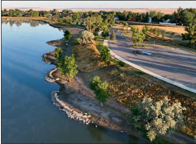
Figure 43. Overview of trail and bank repairs completed at Lake Elmo in April 2022 (photo by Bob Gibson, FWP, Spring 2022).
