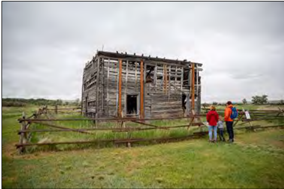
Figure 3. Structure at Gallatin City, within Missouri Headwaters. This structure is threatened due to its deterioration.
