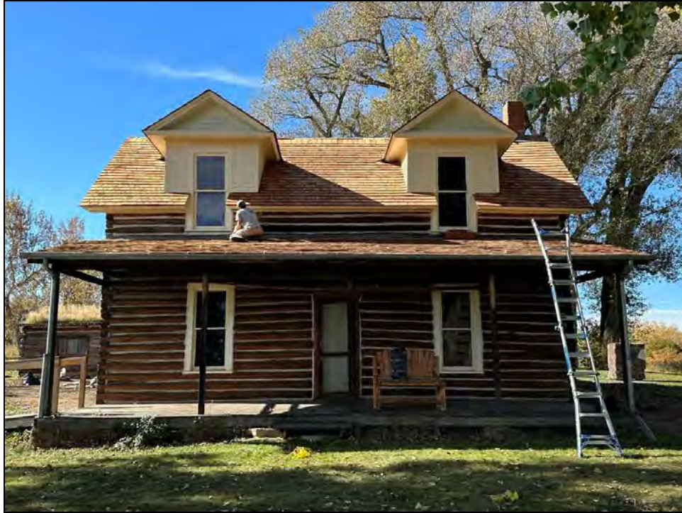
Figure 39. Painting the dormers on the Chief's House, log treatment, and new cedar shingles.
