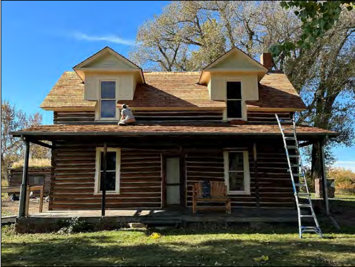
Figure 10. Painting the dormers on the Chief's House, log treatment, and new cedar shingles.
