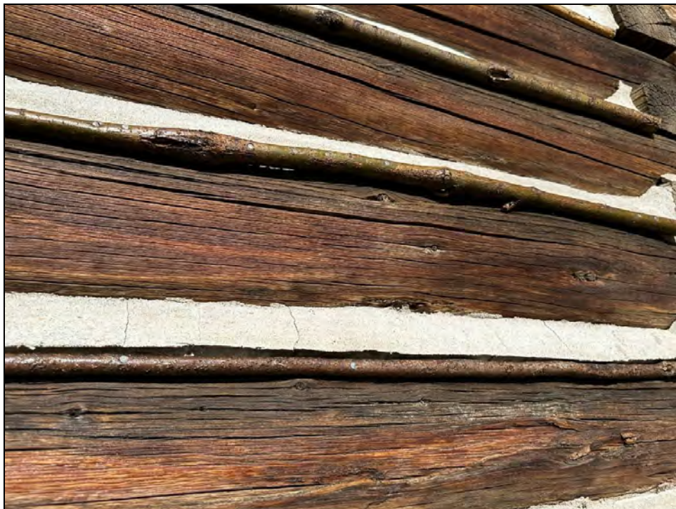
Figure 40. Close up of the replacement willow and treated logs on the Chief's Store.
