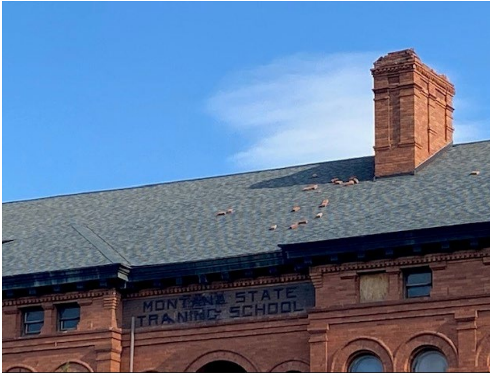
Damage caused by a windstorm in January 2021. The chimney cover was blown off and several bricks have been damaged.
