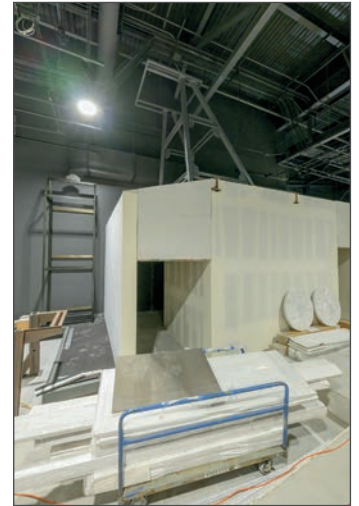
Construction of the Montana Homeland Gallery is in full swing. Here you can see the framing around the steel outline of a headframe that will soon feature an immersive underground mining experience.
