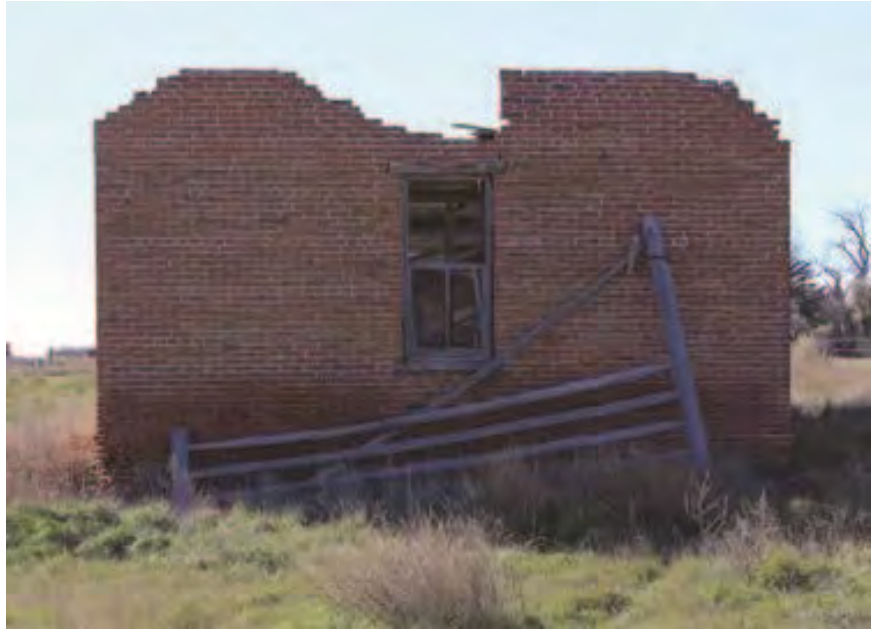
Figure 6: Fort Assinniboine - Field Officers Stable #2. The 2015 storm tore the roof off and the upper portions of the brick walls. Photograph courtesy of the Fort Assinniboine (Boundary Increase and Additional Documentation) nomination, page 107. Photograph taken between October 2015 and June 2016.
