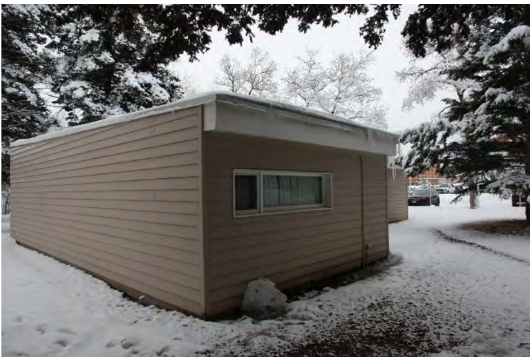
Figure 2: Danforth Chapel, January 11, 2018, at MSU-Bozeman. The wood fascias are wet, causing the paint to flake off. This might be indicative of ice melt getting behind the sheet metal drip cap.
