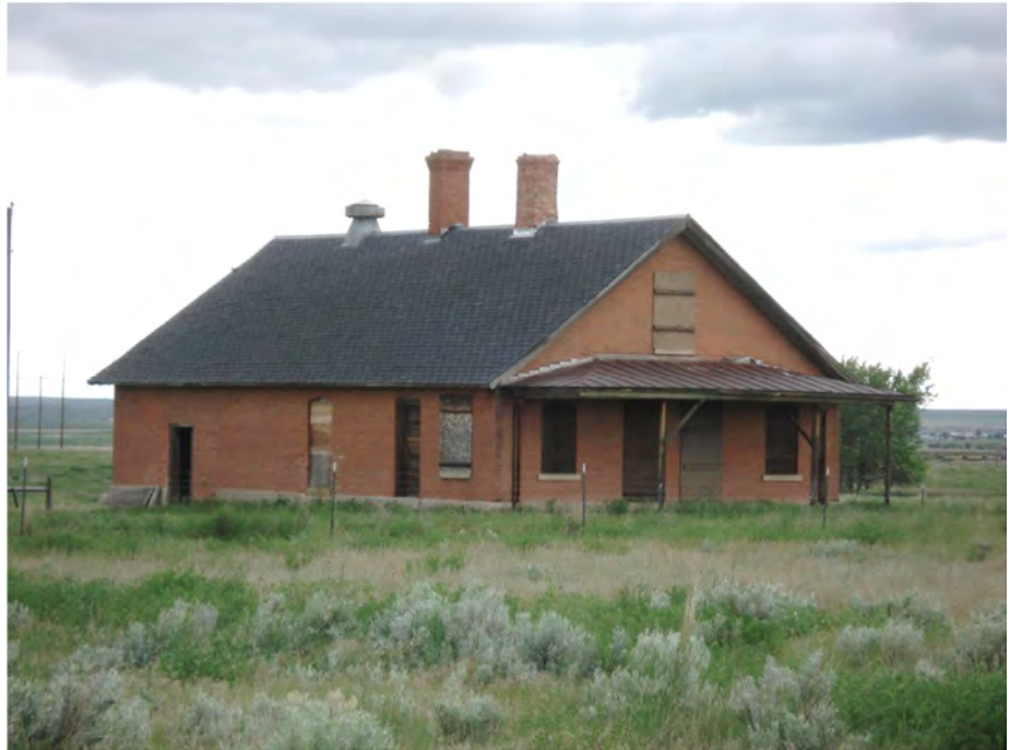
Figure 20: MAES Fort Assinniboine, East Guard House (Building #5418), as maintained in good condition by FAPA.
