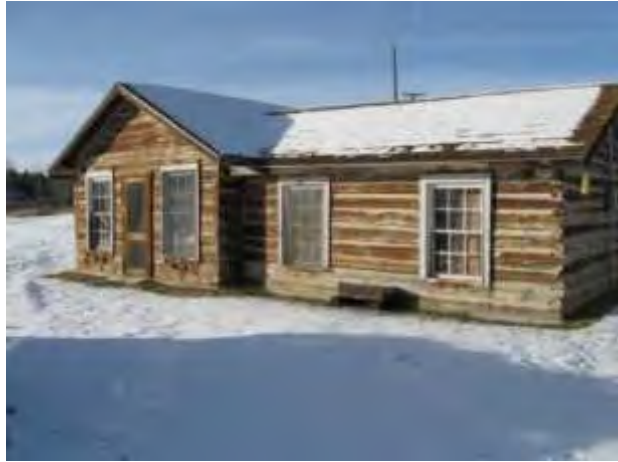
New roof is needed
