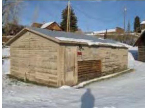
New roof is needed
