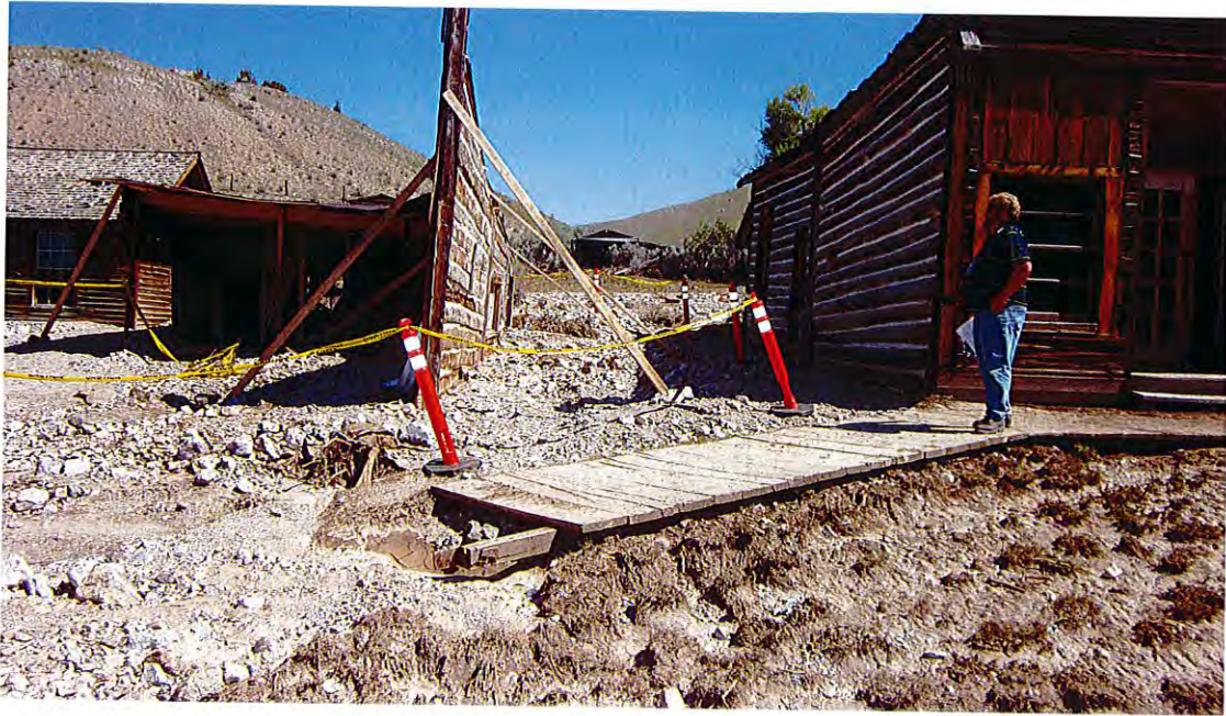
Figure 4. Assay Office (on left) at Bannack NHL damaged by July 17, 2013 flash flood.
